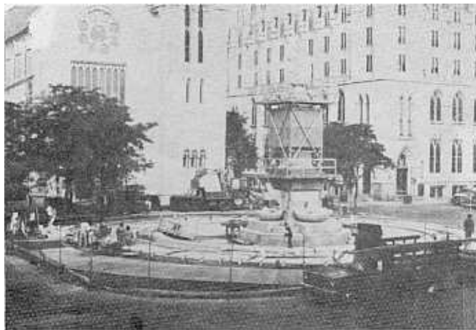
During: Columbus Circle was the recipient of a $200,000 EQBA grant for reconstruction of the 1932 design. Additional monies were raised locally. Photo taken in early October.
